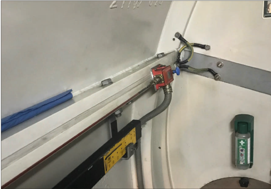
Figure: The basic emergency stops (two blue bottoms) are connected to the red wires following the Nacelle hatch. If stepping up on the hatches it is easy to put a foot on the line and activate the emergency stop.
