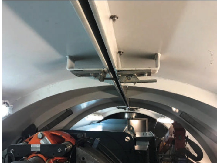
Figure: Location of the two manual locks inside the nacelle.
