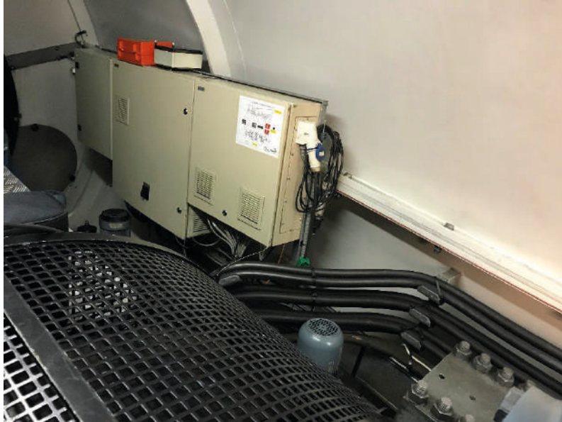
Figure: The multicable is connected under the box to the right
