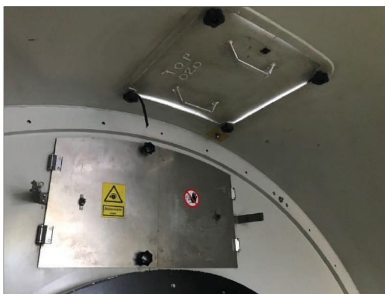
Figure: opening lock to the blades and the small hatch to be opened for a better view when the wind is not in SW.
